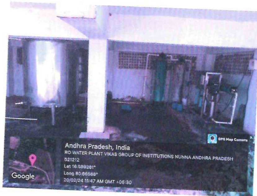
RO PROCESSING UNIT
