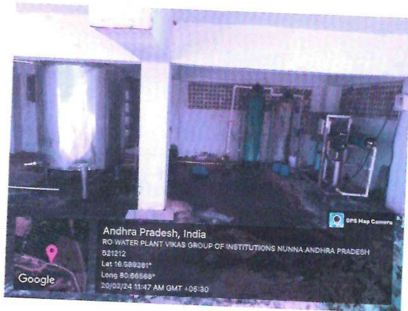
RO PROCESSING UNIT
